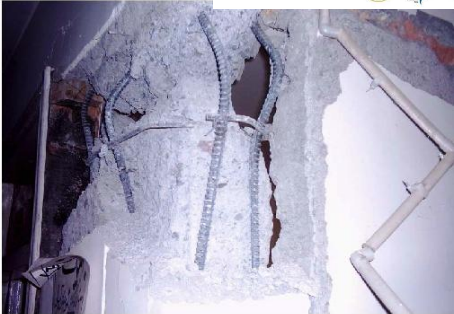
Figure 7: Formation of plastic hinge in the column near the beam-column joint in a UPDRR center building in Mansehra
